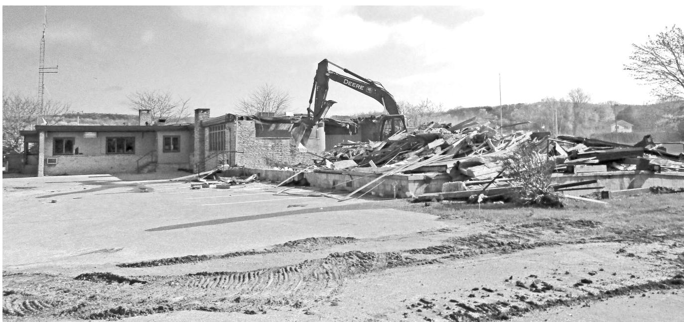
Demolition of Boyne City's long-time city hall began in earnest last week. The 87-year-old building had been home to the city's administrative offices, emergency service departments, MSU extension office and history museum since 1978. Construction of a nearly $7 million new city hall at the same site is set to begin once demolition is complete and expected to take about 15 months. A temporary city hall meanwhile has been set up directly across Lake Street in the Honeywell building.
